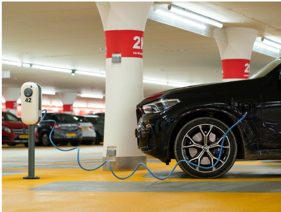
Figure 1-2. Electric Vehicle Charging Infrastructure
