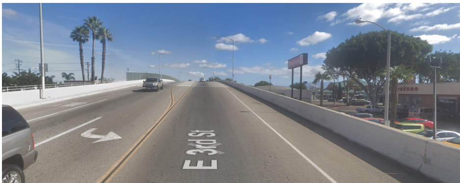
Existing 3rd Street Bridge with Missing Sidewalk on South Side
